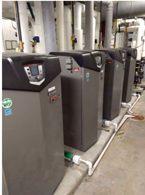
Photograph 5. Natural gas boilers used to heat the Illinois Terminal building.
