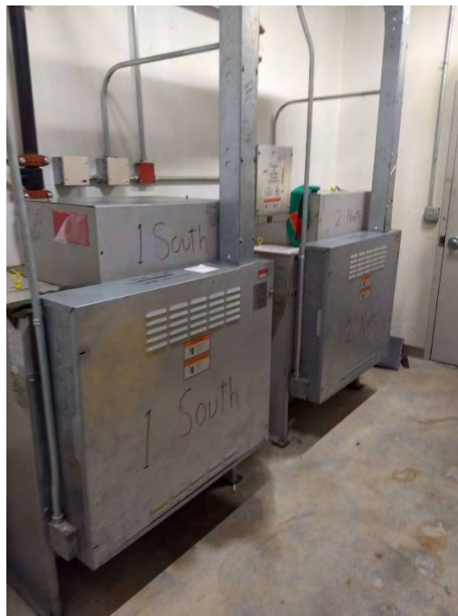
Photograph 6. Machinery responsible for the operation of the hydraulic elevators in the building.
