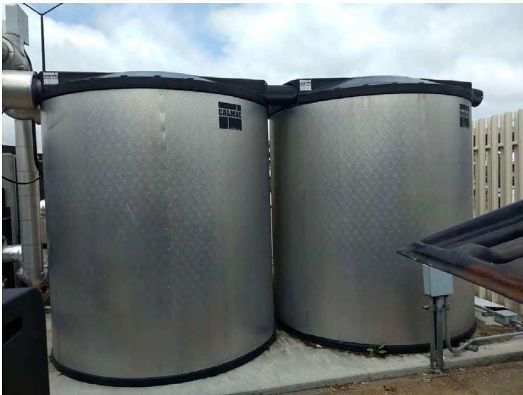
Photograph 8. Ice tanks located in the southeastern corner of the Illinois Terminal.
